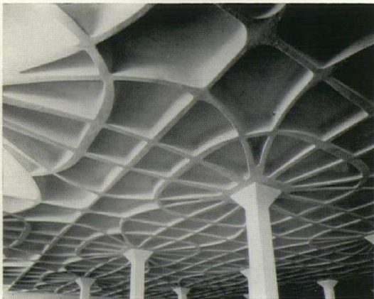
Constructional and static solution - the ribs follow the lines of principal bending moments. The elegance of these lines is not due to the merit of the designer but is a merit of the structure itself.
